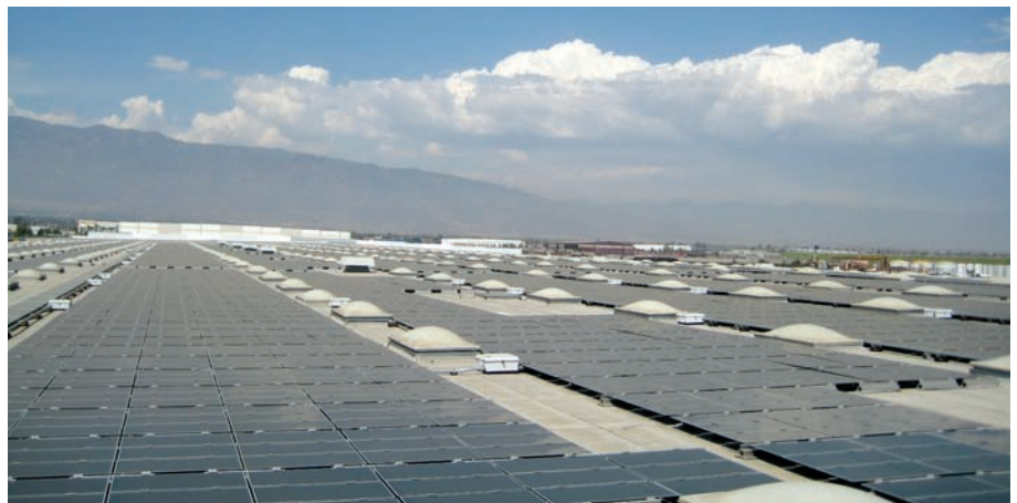
Southern California Edison leased 607,000 square feet of roof space at the Kaiser Distribution Center in Fontana, Calif., to accommodate a 2.4 MW solar installation. Photo courtesy of ProLogis.
