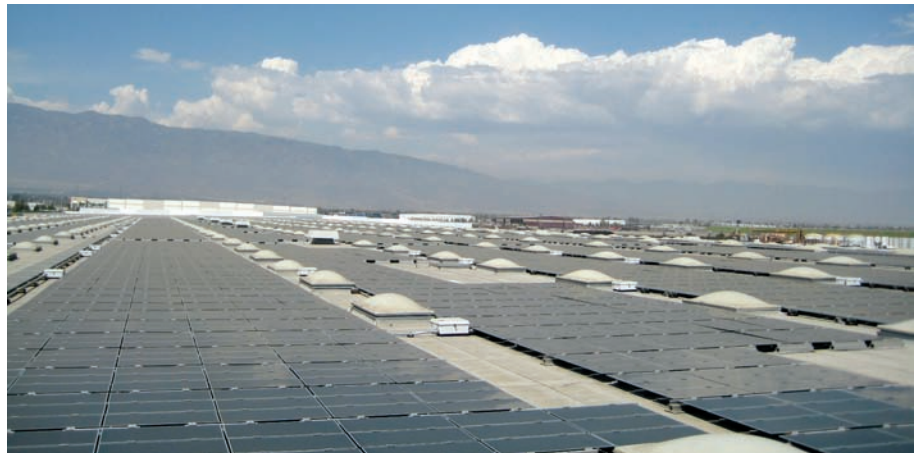
Southern California Edison leased 607,000 square feet of roof space at the Kaiser Distribution Center in Fontana, Calif., to accommodate a 2.4 MW solar installation. Photo courtesy of ProLogis.
