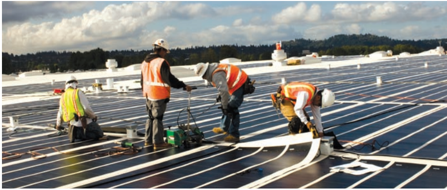
Workers install thin-film solar panels at ProLogis Park PDX in Portland, Ore. Photo courtesy of ProLogis.
